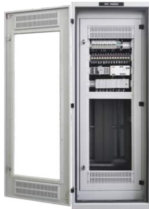
▶ RTU Panosu Remote Terminal Unit Panel
