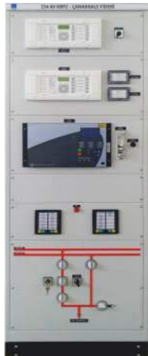
▶ 154 kV Kumanda - Röle Panosu 154 kV Control - Relay Panel
