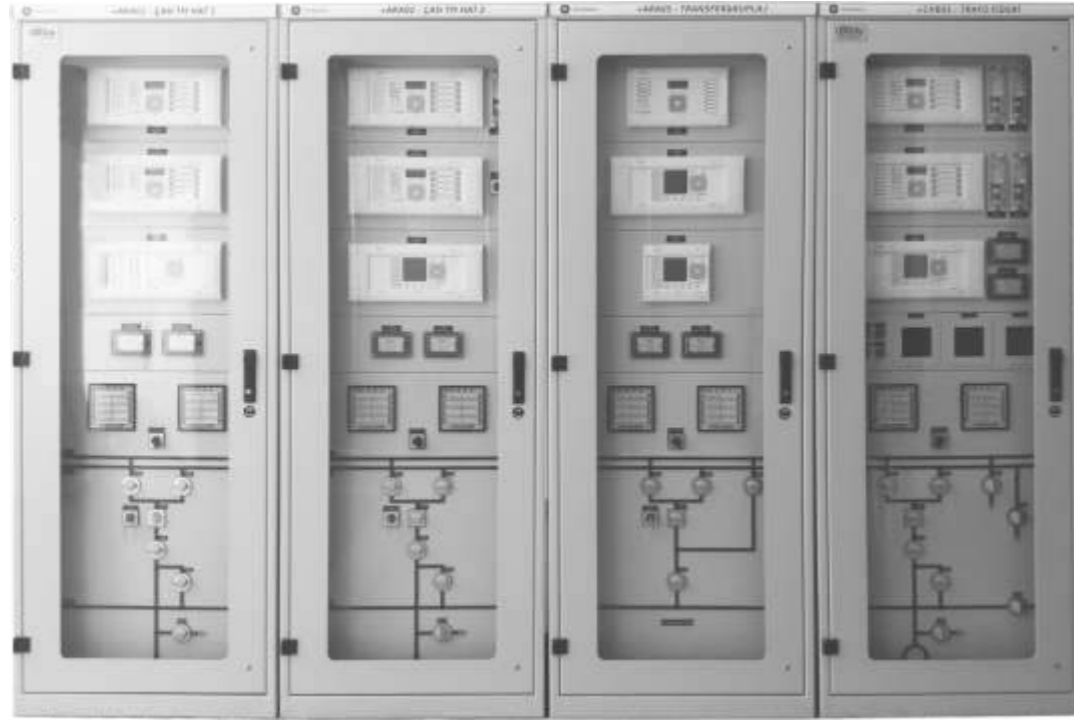
▶ 380 kV Kumanda - Röle Panosu / 380 kV Control - Relay Panel
